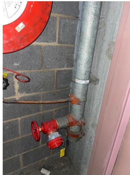
Figure 4: Fire hydrant in cupboard.
