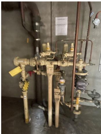
Existing High pressure gas boundary regulator.
