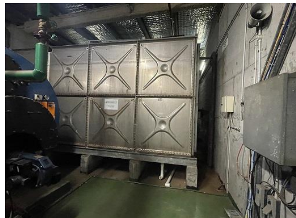
Existing Combined CW. & FH water storage tank.
