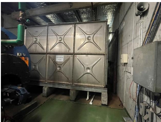
Figure 5: Roof top combined potable/fire hydrant tank.
