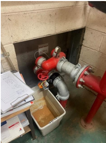
Figure 1: Existing fire hydrant booster assembly
