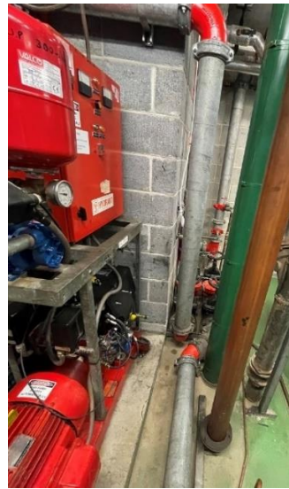
Figure 2: Existing Diesel/Electric Hydrant pump
